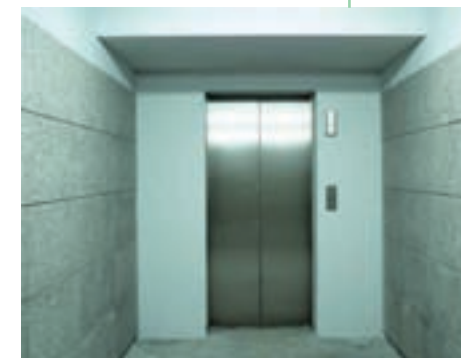
HIGH-TECH ELEVATORS WITH GENERATOR BACK-UP
